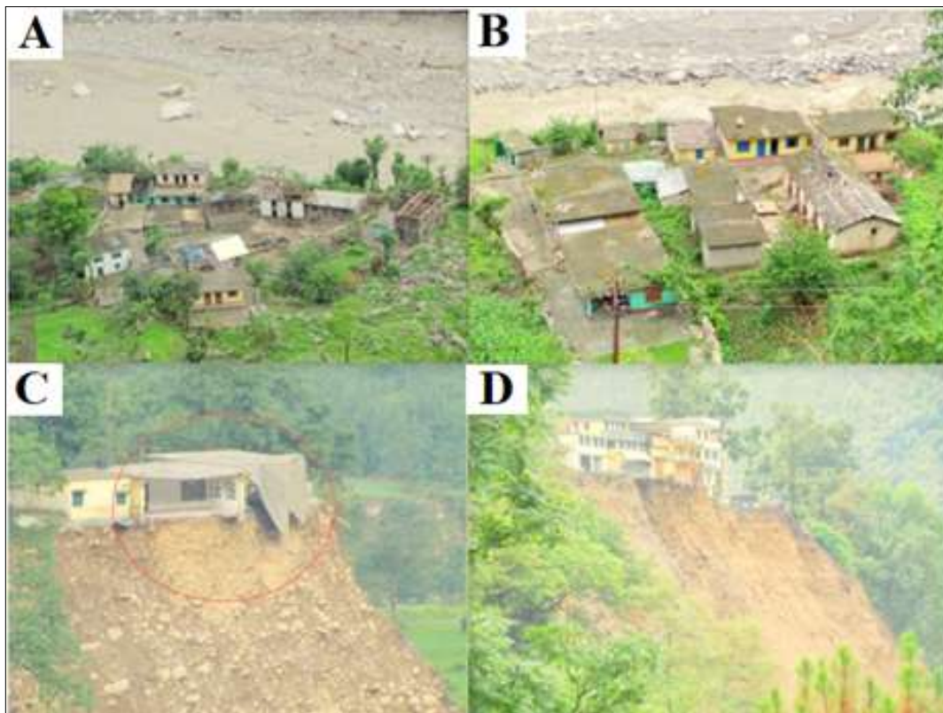
Plate 1: Damaged houses in Gori Ganga watershed: (A) at Umargada village in 2019, (B) at Balibagar village in 2019, (C) school building at Madkote village in 2013 and (D) at Madkote village in 2013.
