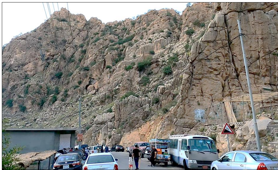
Fig 4: The risk of rock masses exposed to collapse on the road.
