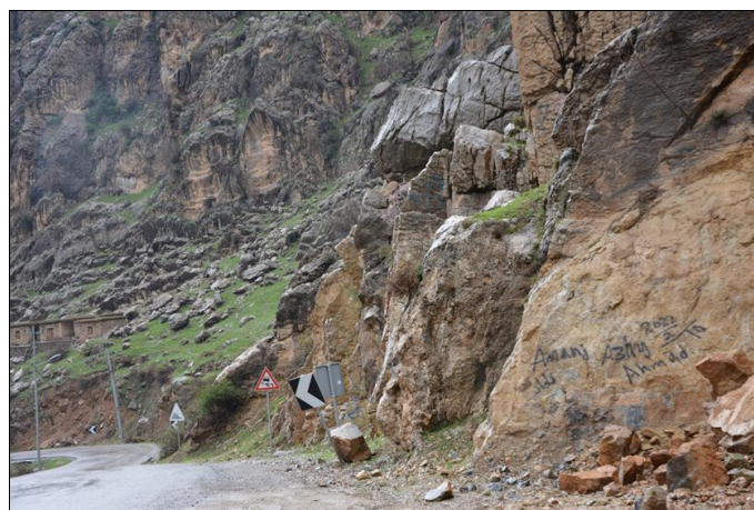
Fig 2: Shows an overall view of the slopes, the width of the paved road, and the absence of a ditch for rockfall
