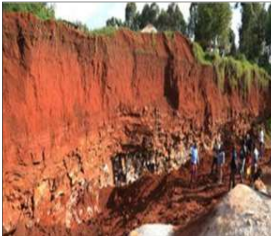
C. Loose Topsoil and Soapstone Rocks
